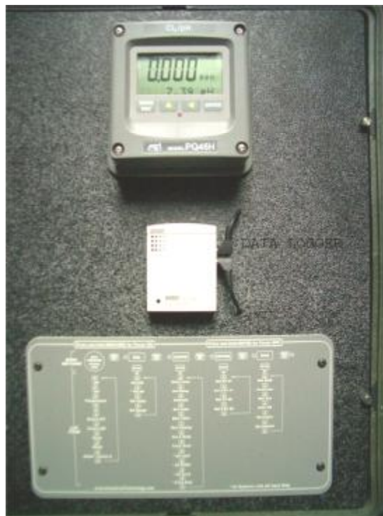
Figure 2 - Front View of Hinged Panel
