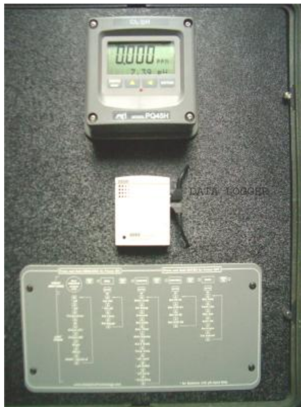
Figure 2 - Front View of Hinged Panel
